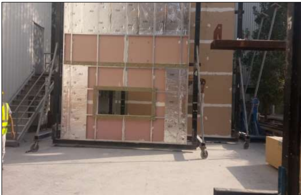
Picture 4: The cavity fire barrier and mineral wool slab were fixed using grip nails on the base wall.
